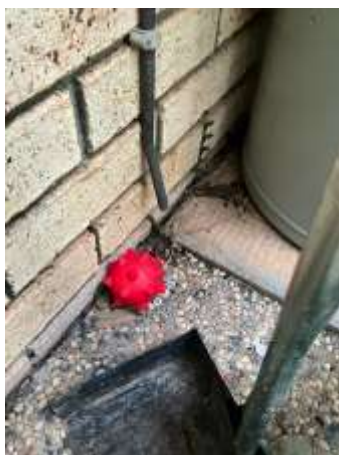
The presence of excessive moisture
