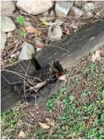
Wood rot/fungal decay to fence - to avoid further deterioration recommend engaging a fencing contractor to repair/replace
