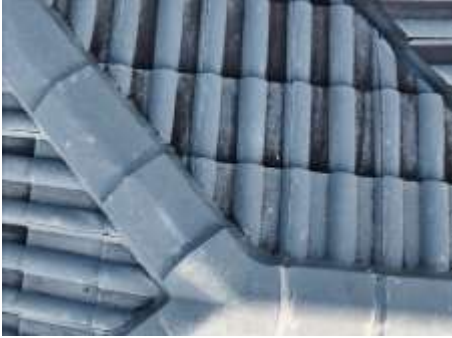
Cracked tiles and Missing/cracks to the pointing, recommend engaging a roofer to rectify and reduce the risk of water penetration into the building.
