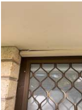
Sagging visible to the external soffit boards at the front elevation/ separation
