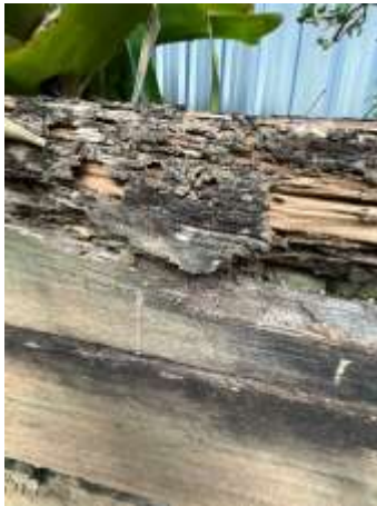
Termite workings and damage to the boundary fencing. Recommend replacement to affected ares and treatment to eradicate Termite colony.
