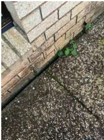
Side yard concrete slab been shifted, signs of subsidence and movement, inconsistent gap visible. Recommend engaging a licensed Builder for further assessment and repair proposals.
