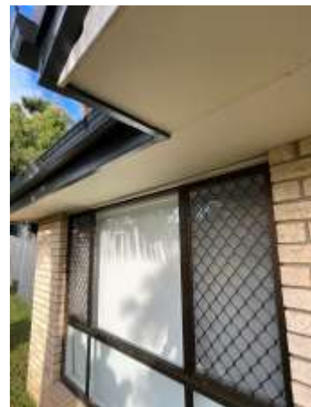
Sagging visible to the external soffit boards at the front elevation/ separation
