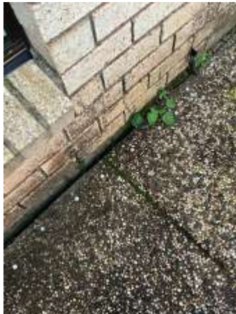
Mould cleaning recommended from the external bricks
