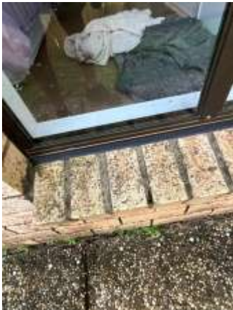
Mould cleaning recommended from the external bricks
