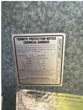
The previous termite management system stickers - please contact the installer
