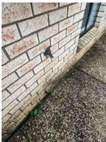
The presence of excessive moisture
