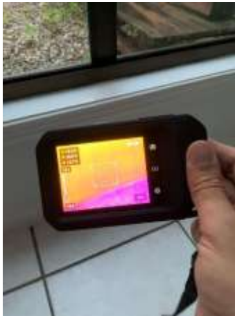
High moisture readings to internal walls. Invasive investigation recommended by a Licensed Builder to ascertain source of leak/moisture and to determine if there is any concealed damage to timber frames and other elements.
