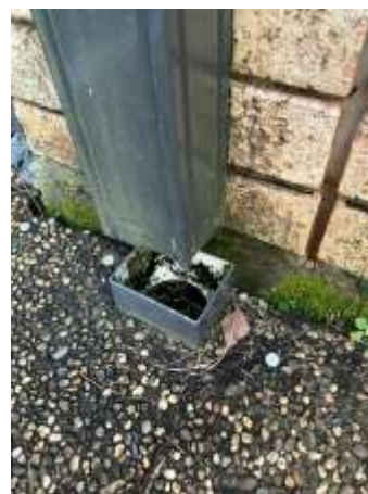
The presence of excessive moisture
